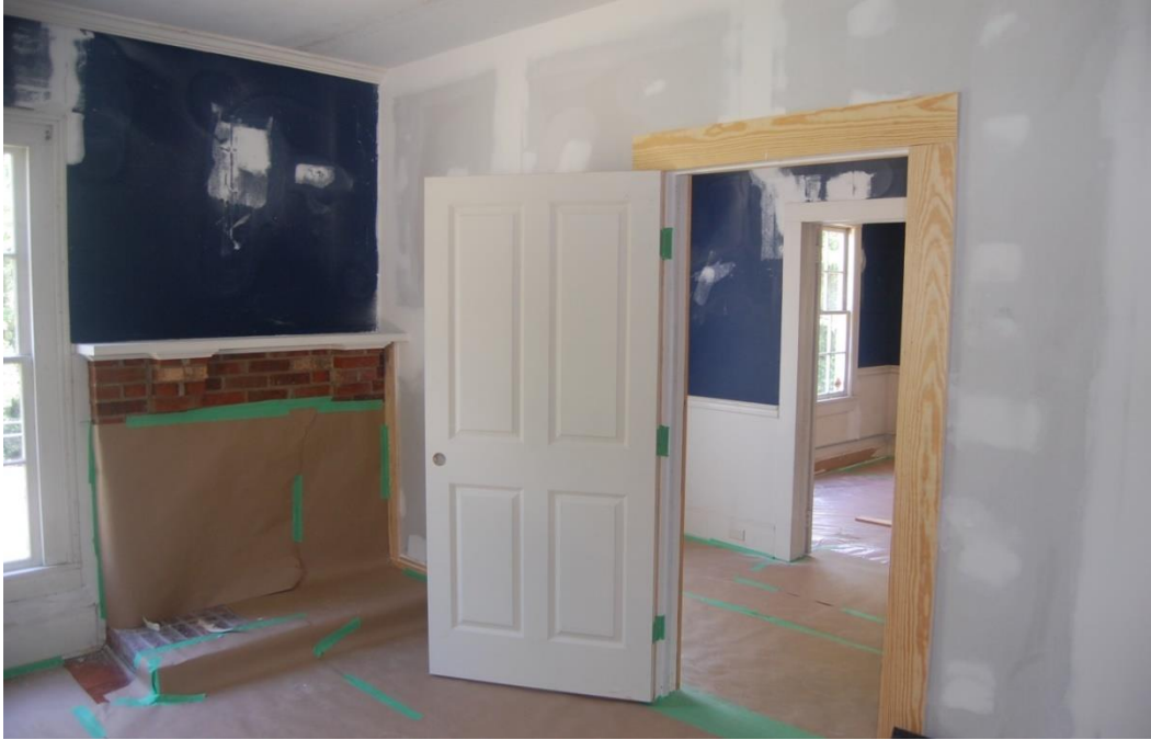
Harkey-McEwen-Moore House, After Relocation, 2016, Interior, North Room of Main Block, Showing Fireplace Mantel and Modern Partition Wall, Looking into Rear Ell Dining Room.
