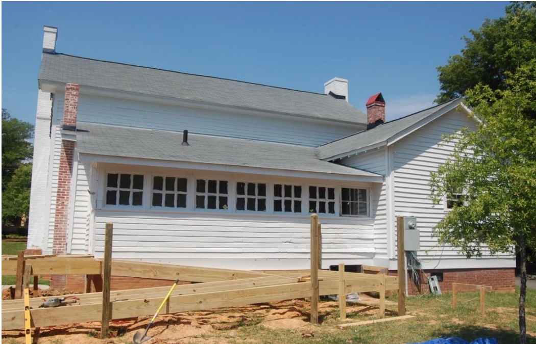
Harkey-McEwen-Moore House, After Relocation, 2016, Rear (East) Elevation, Showing Ramp Under Construction and Outbuilding on Right, Looking North.
