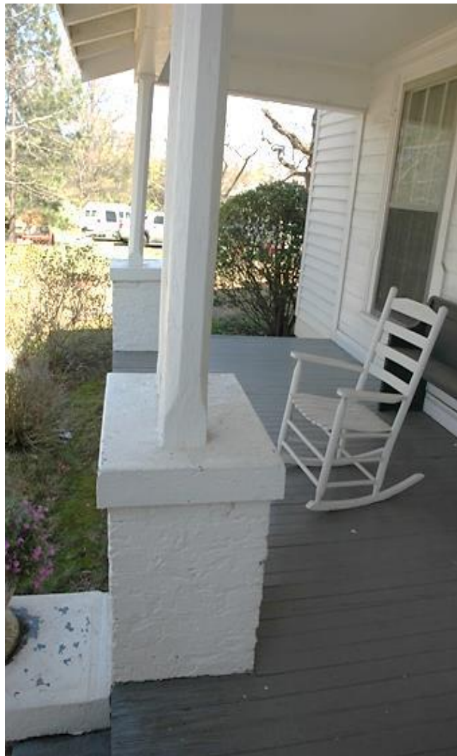
Harkey-McEwen-Moore House, Before Relocation, 2009, Porch Posts. (Source: Charlotte-Mecklenburg Historic Landmarks Commission Files)
